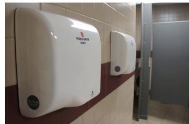
ADA SLIMdri in one of the Men's room
